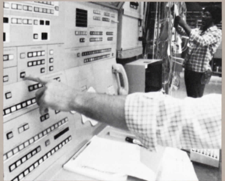
Below—One of the biggest R and D programs of all time was mounted by the Bell System for the introduction of electronic switching into the network. This is the console of the first ESS, Succassunna, N.J. in the spring of 1965.
