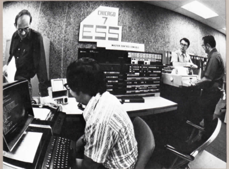
Western's electronic switching system for long distance calls, the #4 ESS, was our first digital switcher. The first installation was in Chicago. Rapidly, the 4E began to replace the #4 crossbar offices nationwide.
