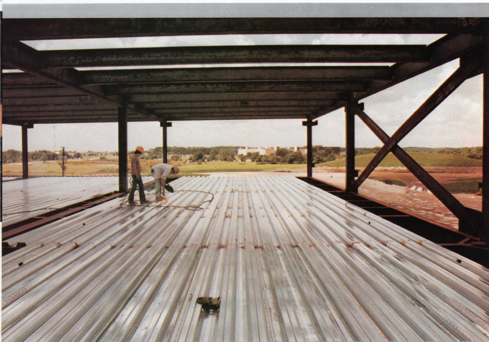
Following official groundbreaking ceremonies in 1979, workmen began positioning steel framework (left and above) in April at the site of the company's new Software Center in Lisle, Ill.
