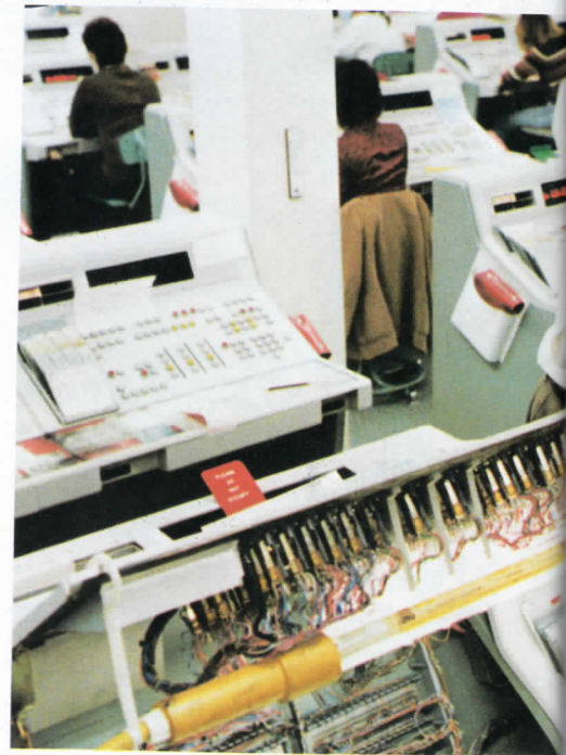
Top — Tony Severini explains crossbar wiring procedure to newcomer Barbara Murphy. Below — Joe Roche checks modification of N.J. Bell operator's position with installer Bill Tharp.
