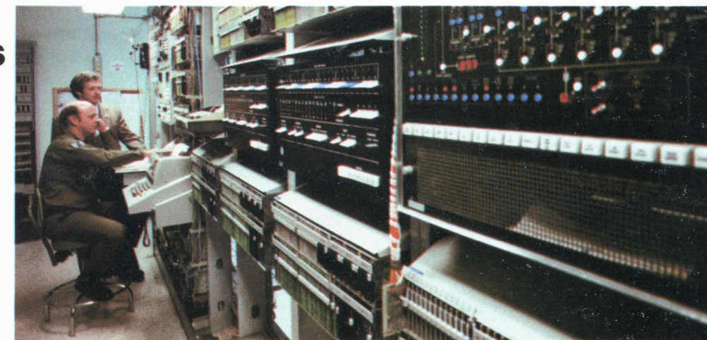
At Edwards Air Force Base in the Mojave Desert we turned over an electronic switching system for use as a customer-owned and maintained base communications system.
