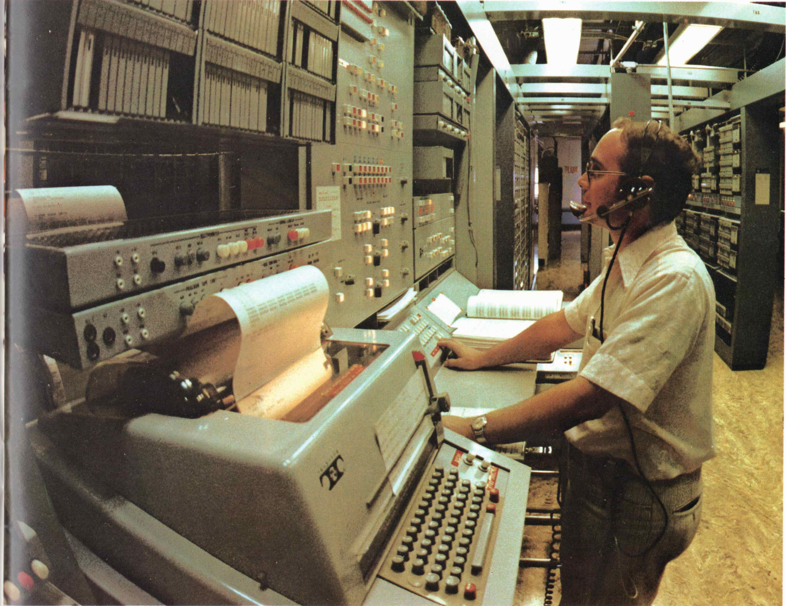
Bottom Right: A telephone company craftsman operates the console of this electronic translating system which permits Common Channel Interoffice Signaling—a new high speed way of making long distance connections.
