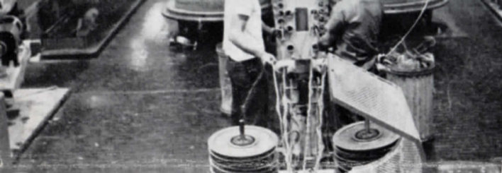
DENNIS KARLOFF and JIM FOX, 253, in preparation for running a 600 pr. cable, thread the stranding cabler with multi units of 50 prs. of wire each.
