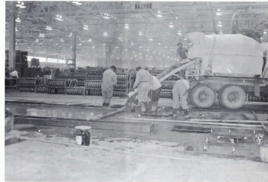
Cement is poured before installation of new machinery in the Cable Plant. This new addition will be the June production feature.
