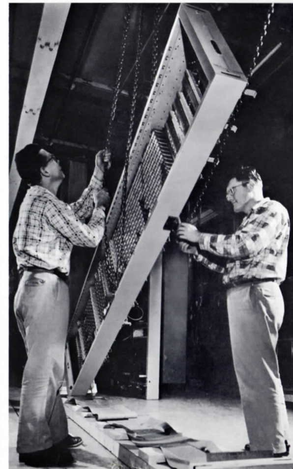
W.E. installers at work in a new central office installing W.E.-made equipment for a Bell System operating company
