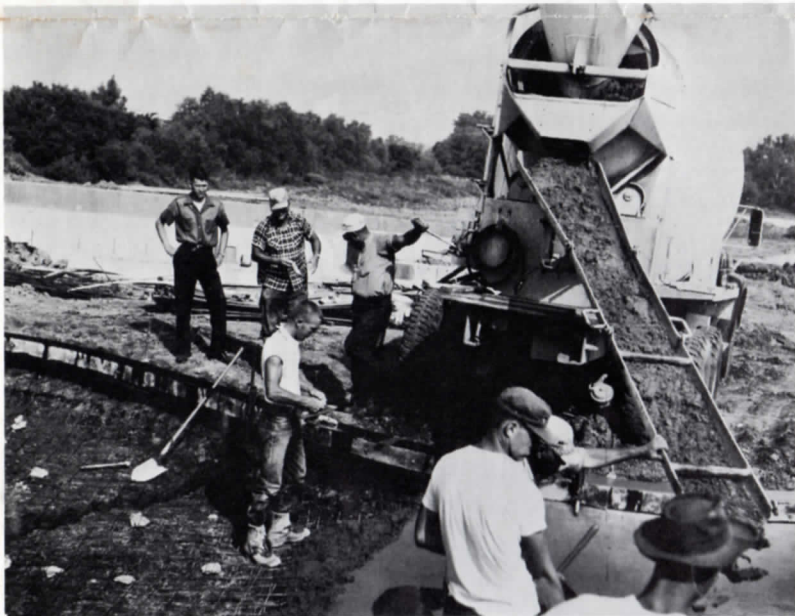
Dave Van de Water, at left, watches the pouring of the wading pool.
